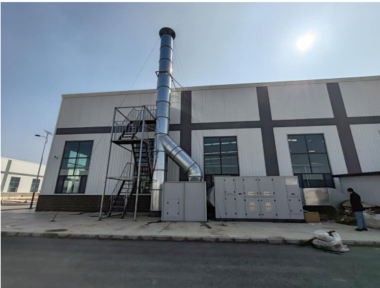
“UV 光解+活性炭吸附”装置+15m 排气筒
